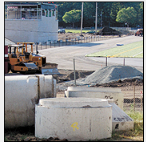
Construction work continues on Reading Memorial High School, with work in progress seen here around the new football field. - Staff photos by Mac McEntire
