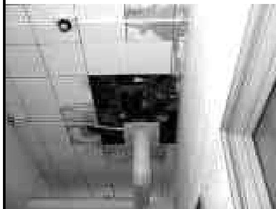
One of dozens of water damaged and collapsing ceiling tiles throughout the school.
